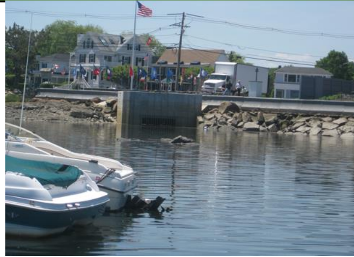
Tide gate (TG) located at Border Street.
